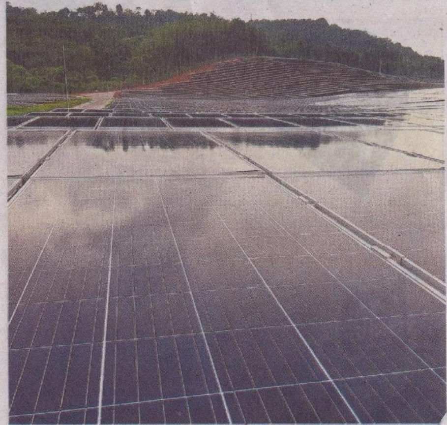
Power generation: Leader Energy's RM180mil solar power project in Kedah
